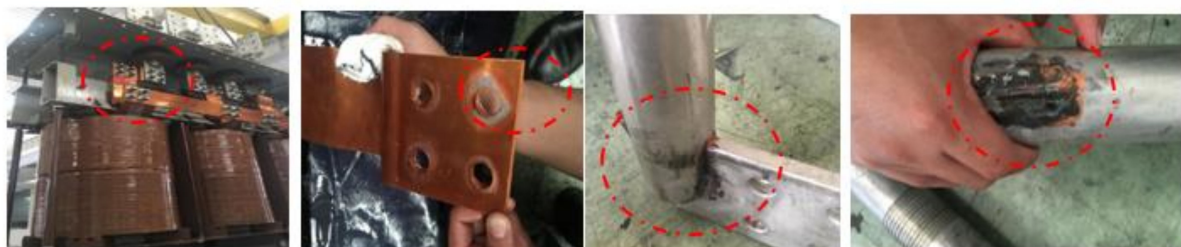
Figure 11. Arcing due to loosened bolts and nuts inside TR2, 22 kV/416 V, 3 MVA.
