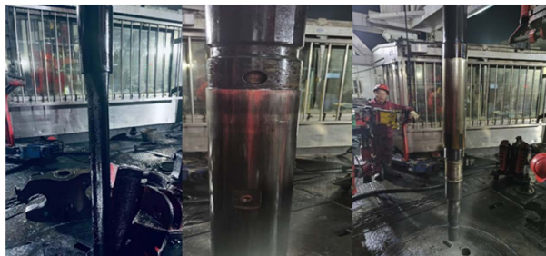
Figure 4. Outlet pipe, RD valve, CQ-CPV valve.
