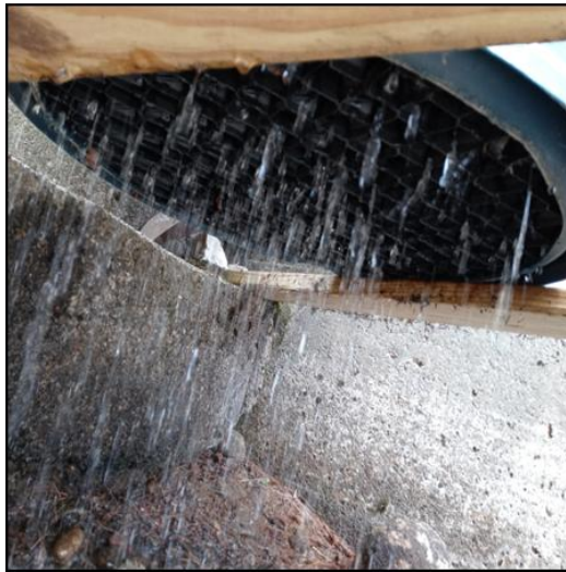
Fig. 4. Bio-tower CF-1900 water Distribution [27]
